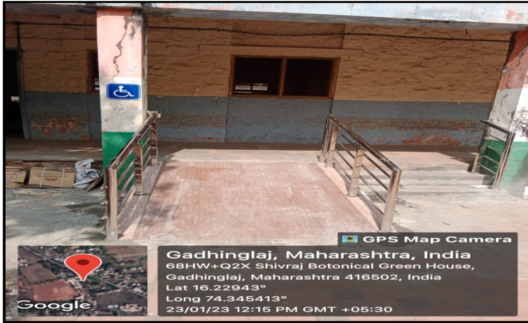
Ramps for Divyangjan
